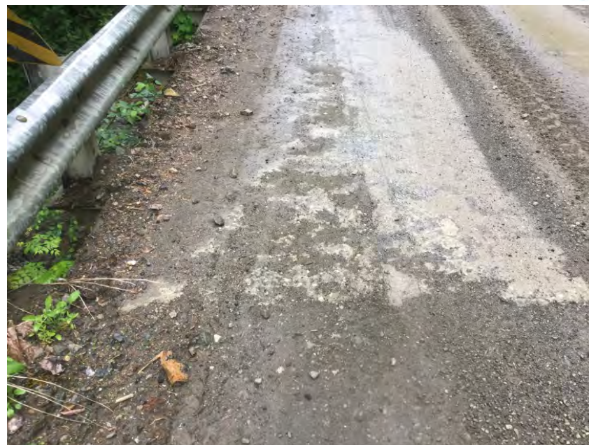
Significant surface damage at left approach - no sign of damage to underside of slabs
