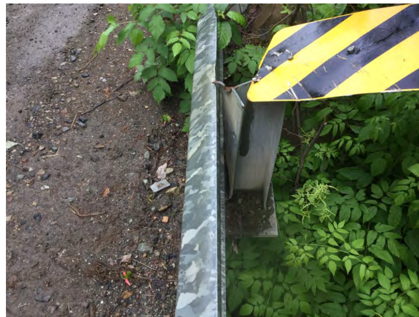
Damage to upstream right bank riser
